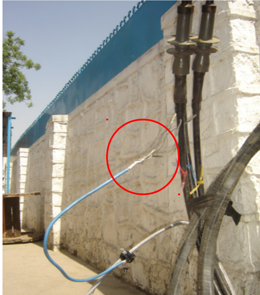
Earthing in HVDS
