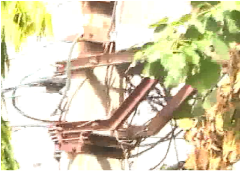
High Voltage Distribution System
